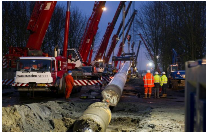
District Heating, e.g. Leiding over Noord
